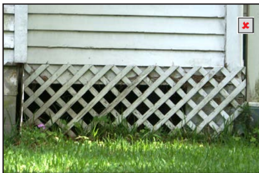
Incompatible lattice panel placement
