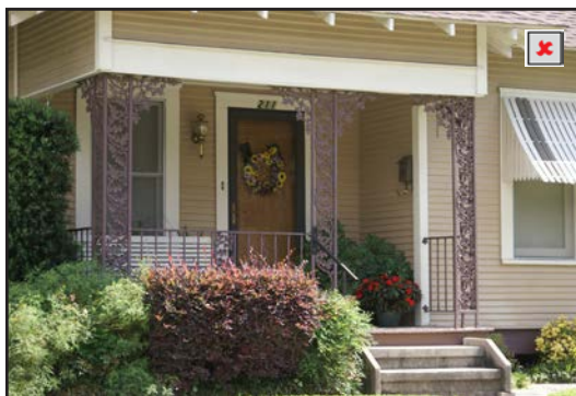
Incompatible metal replacement posts on a Craftsman house
