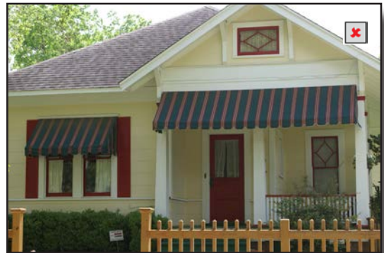
Incompatible fabric awnings over window and porch
