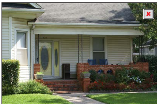
Incompatible brick railing and metal posts on a Queen Anne house
