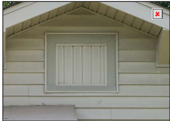
Incompatible gable window or vent covered with siding
