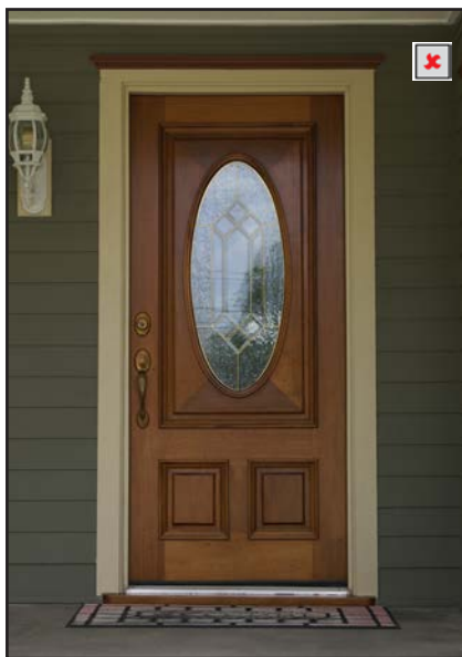
Incompatible replacement front door
