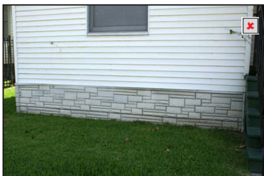
Incompatible faux stone foundation skirting
