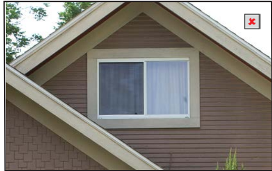
Incompatible replacement gable window
