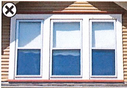
Unfinished metal windows such as these alter the character of window openings, and should not be used in highly visible locations.
