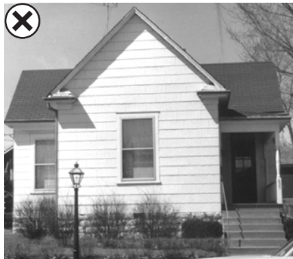
Before: A historic house with inappropriate synthetic siding
