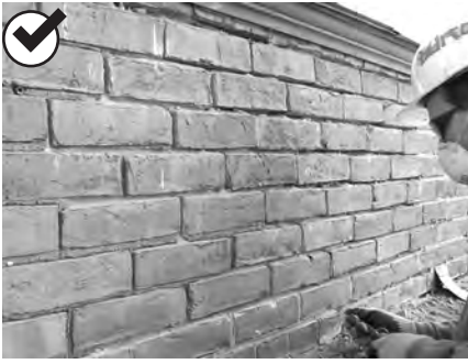
Re-point mortar joints where there is evidence of deterioration.
