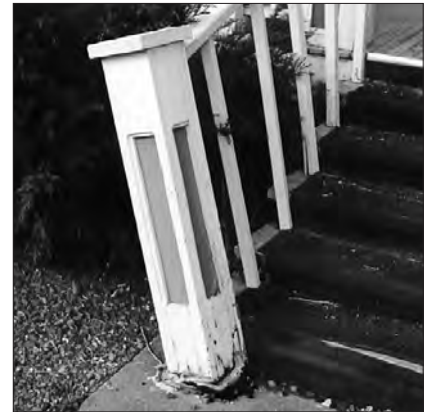
Before: A deteriorated handrail.
