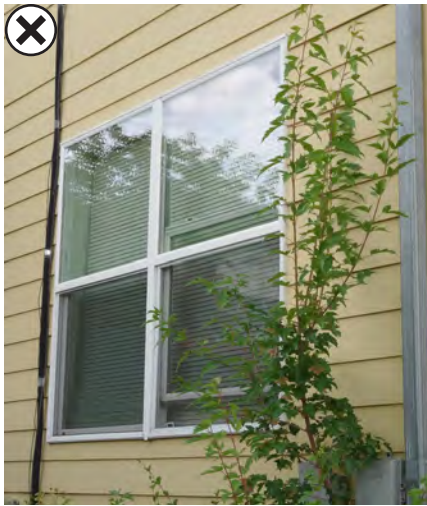
The profile of this window and its trim both lack the proper depth.
