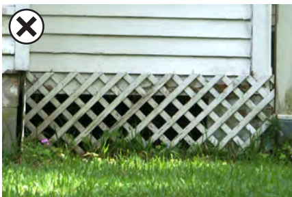
Examples of Inappropriate unframed lattice
