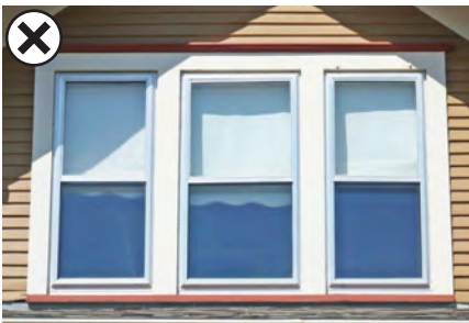
Unfinished metal windows such as these alter the character of window openings, and should not be used in highly visible locations.
