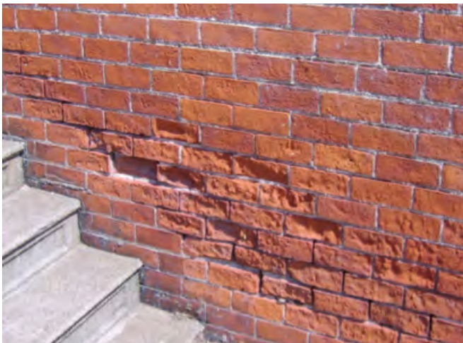
Brick showing damage from inappropriate cleaning (photo courtesy of Heritage Ohio)
