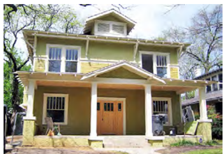
Reconstruction of the porch on a historic house: (top) before; (bottom) after
