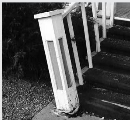
Before: A deteriorated railing should be repaired when feasible.
