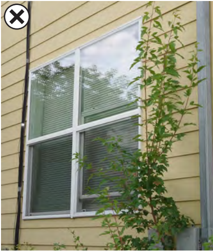
The profile of this window and its trim both lack the proper depth.
