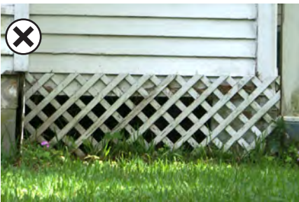
Examples of inappropriate unframed lattice
