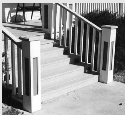
After: Railing has been repaired and the base of the post has been replaced in-kind.
