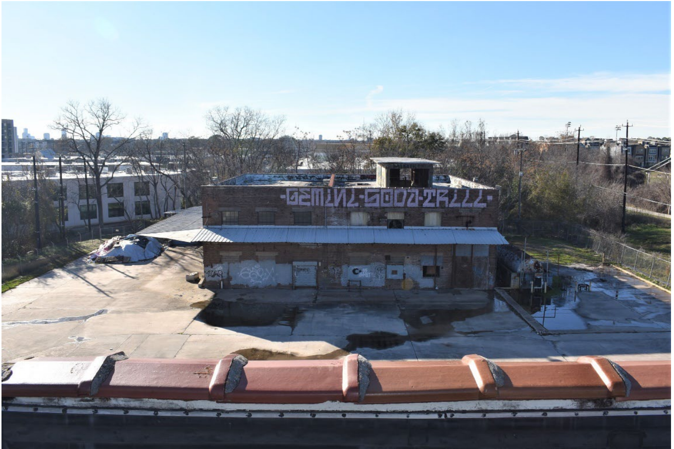
Photo 8 Boiler and Engine House; East elevation; view from roof (rear) of main building, west
