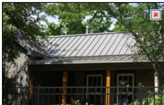
Incompatibly scaled metal roof
