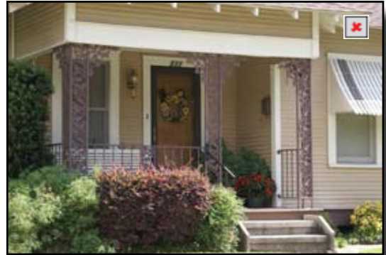
Incompatible ornamental metal replacement posts on a Craftsman house; these would be compatible with a Minimal Traditional house
