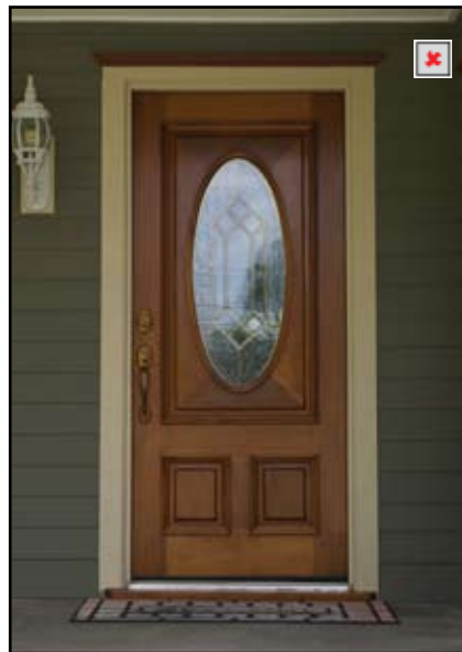
Incompatible replacement front door
