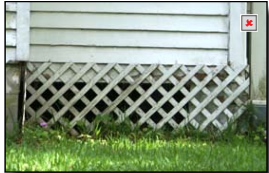
Incompatible lattice panel placement overlapping siding
