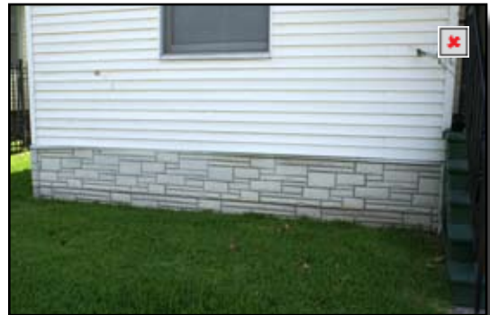
Incompatible faux stone foundation skirting
