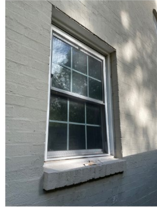
D1 - EXISTING: Non-original window on west elevation facing Woodhead Street. Added during 1977 renovation of kitchen.
