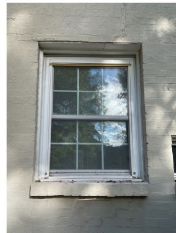
D2 - EXISTING: Non-original window on west elevation facing Woodhead Street. Added during 1977 renovation of kitchen.
