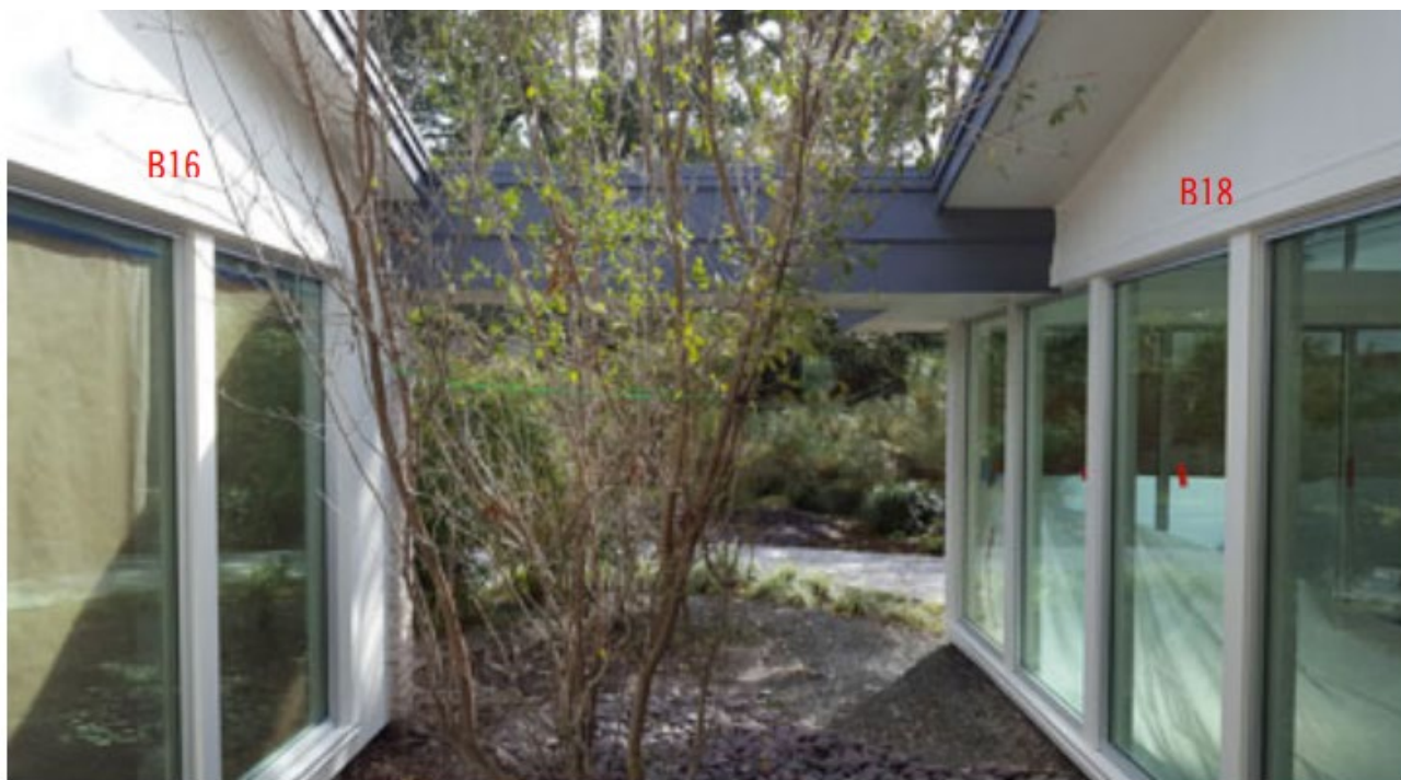
10 – Rear Courtyard, facing North towards backyard – showing typical window conditions of B16 and B18
