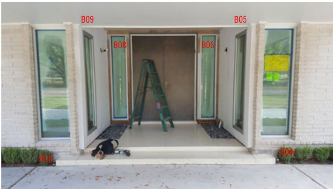
09 – Front Entry at North Elevation – showing typical brick and wood cladding conditions of windows B04~B10
