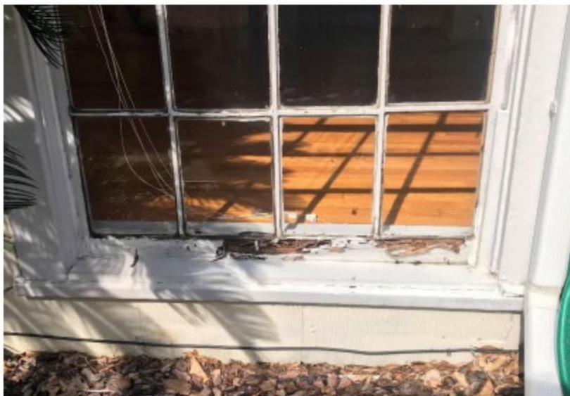
Figure 9 WINDOW F1: Rotten Frame
