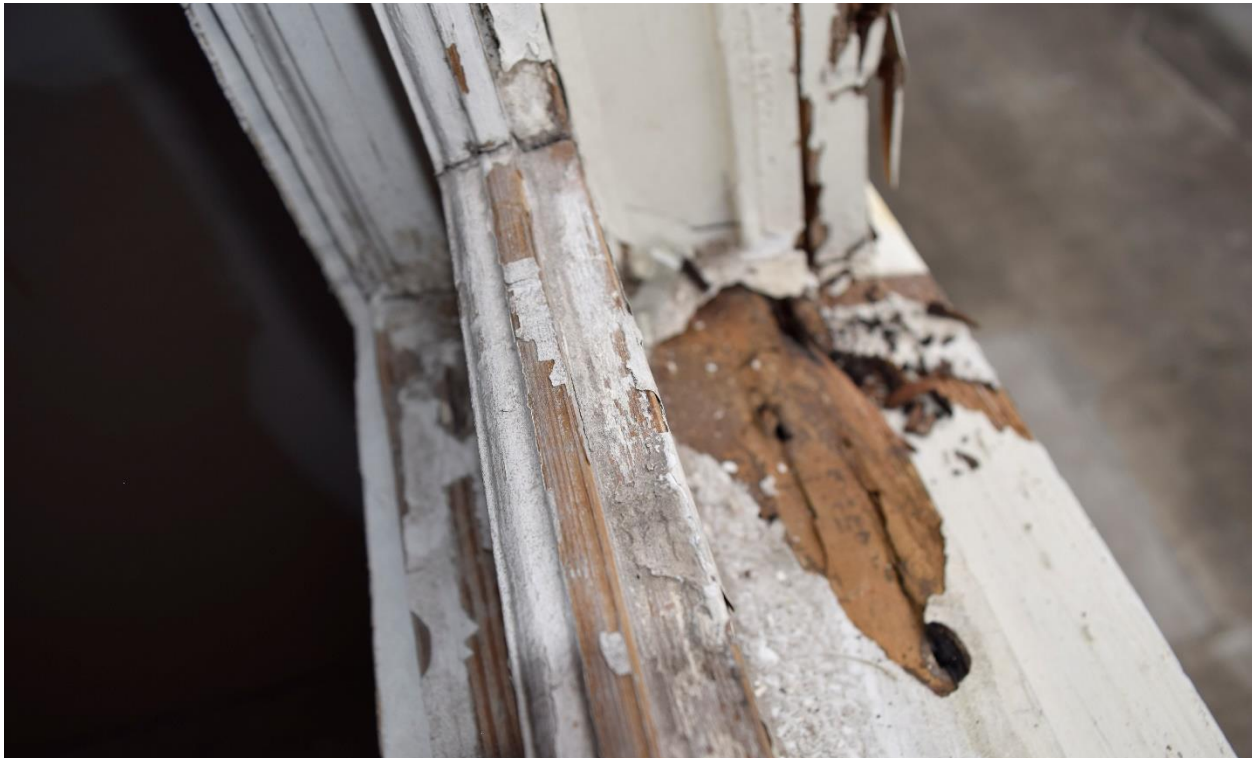
Upper-floor window to be replaced on West Elevation due to wood rot
