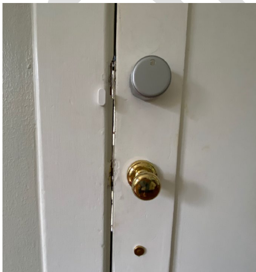
GAP IN LOCK – SAFTELY CONCERN OF APPLICANT
