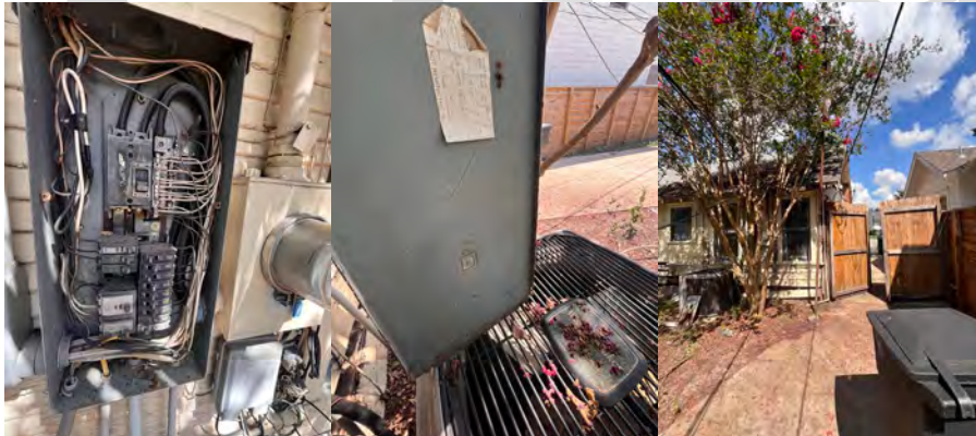
The subject property includes the electrical panel, service lines, and condition of breakers.
