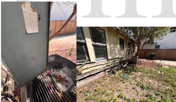
HVAC system for the subject property
