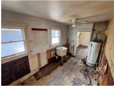
Kitchen area with nonfunctional water heater.
