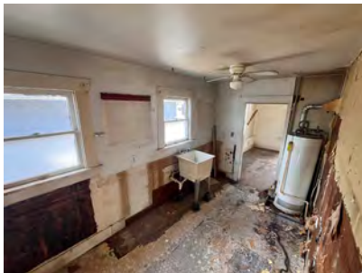
Kitchen area with nonfunctional water heater.
