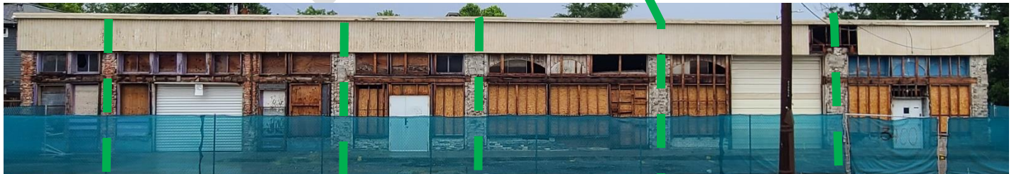
Front (South) elevation as seen by public, agent, owners, staff, and commission members at special meeting held on site, September 19, 2023.
