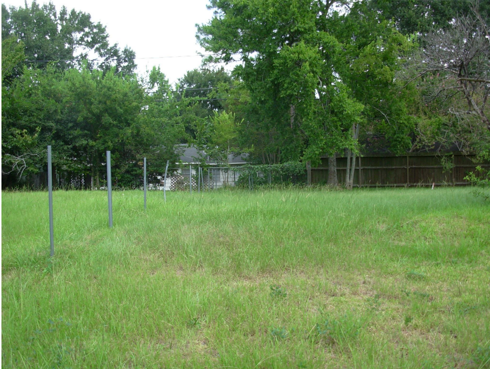
Photo 5. View looking north of possible fault scarp locates southeast corner of Westview and Bunker Hill Road. Photo was taken on the downthrown and upthrown is on the top side of the photo.
