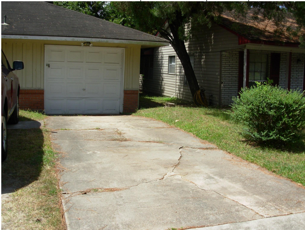
Photo 6. View looking south of possible fault scarp on Westview Drive. Photo was taken on the upthrown side of fault. The ground elevation at the garage door is lower than where the truck is parking.
