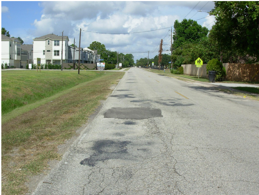
Photo 4. View of general pavement conditions along Neuens Road.
