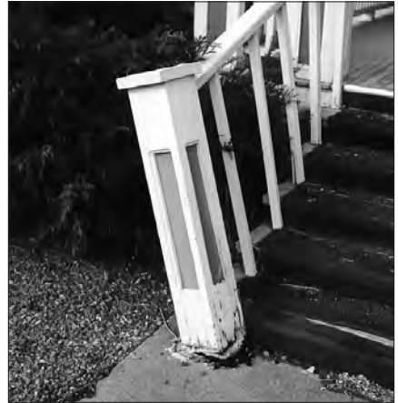
Before: A deteriorated handrail
